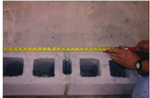
Then measure 1200 along the other side and mark the brick or block.
