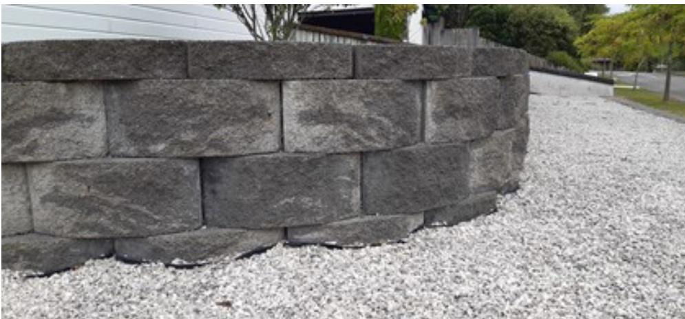
Keystone wall with internal fibreglass rods to keep individual stones in position.
